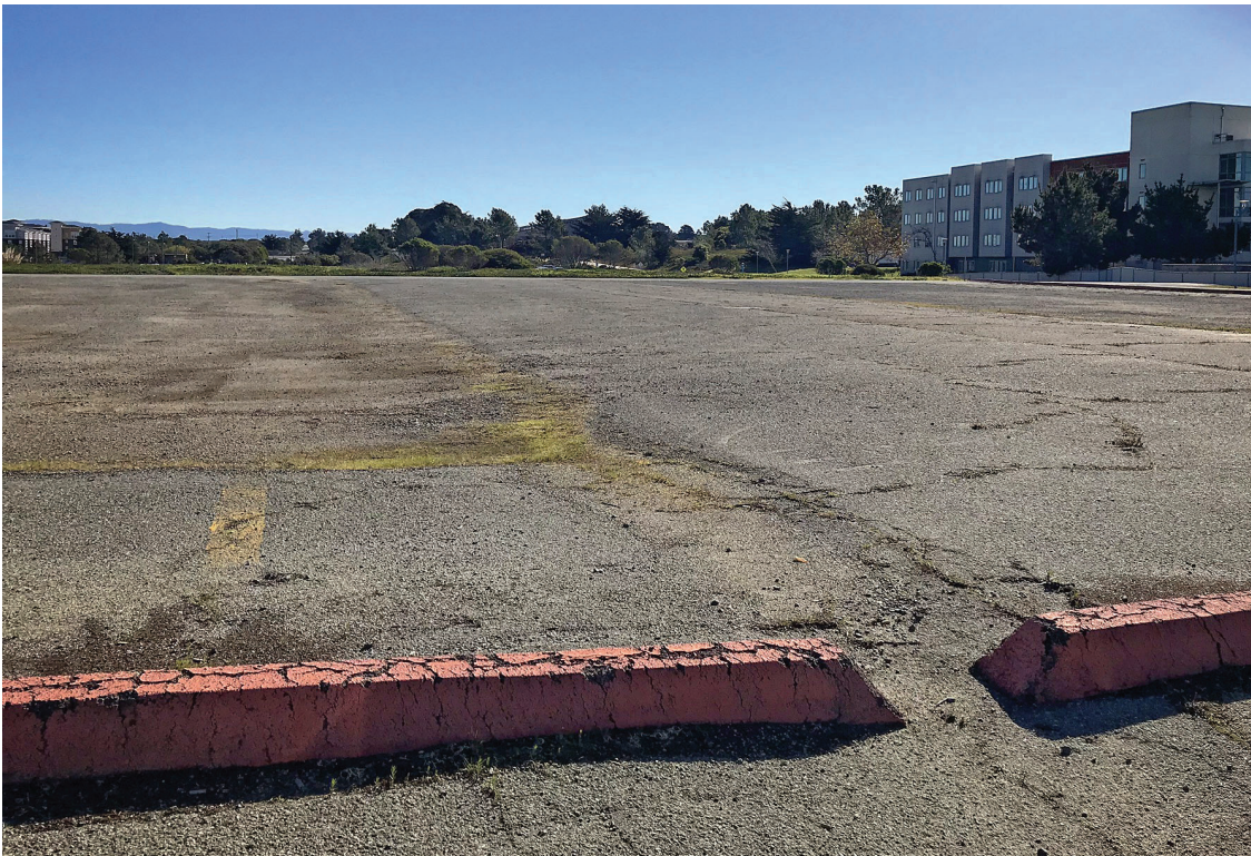
Deteriorated pavement area with views of Promontory Student Housing (far left) and North Quad Housing (far right)
